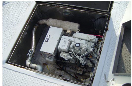
IN BOW 6.5KW DIESEL GENERATOR
